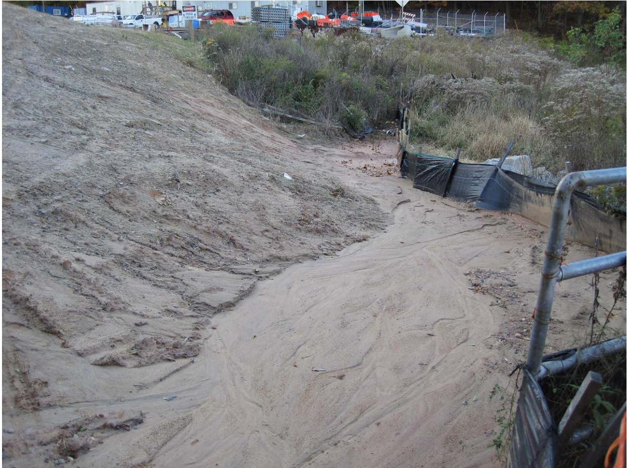
495 Hot Lanes construction mud piling up on the banks of Accotink Creek, on its way to the lake.
