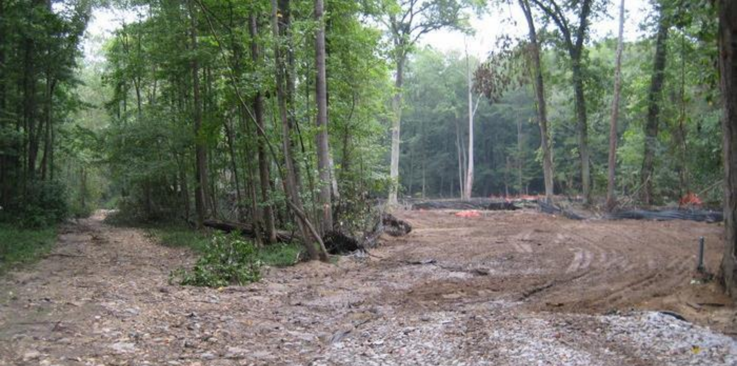
Building of the Cross County Trail, Fairfax County; permanent trail (right) and temporary staging area (left) at north bridge site (Sept 10, 2008)
