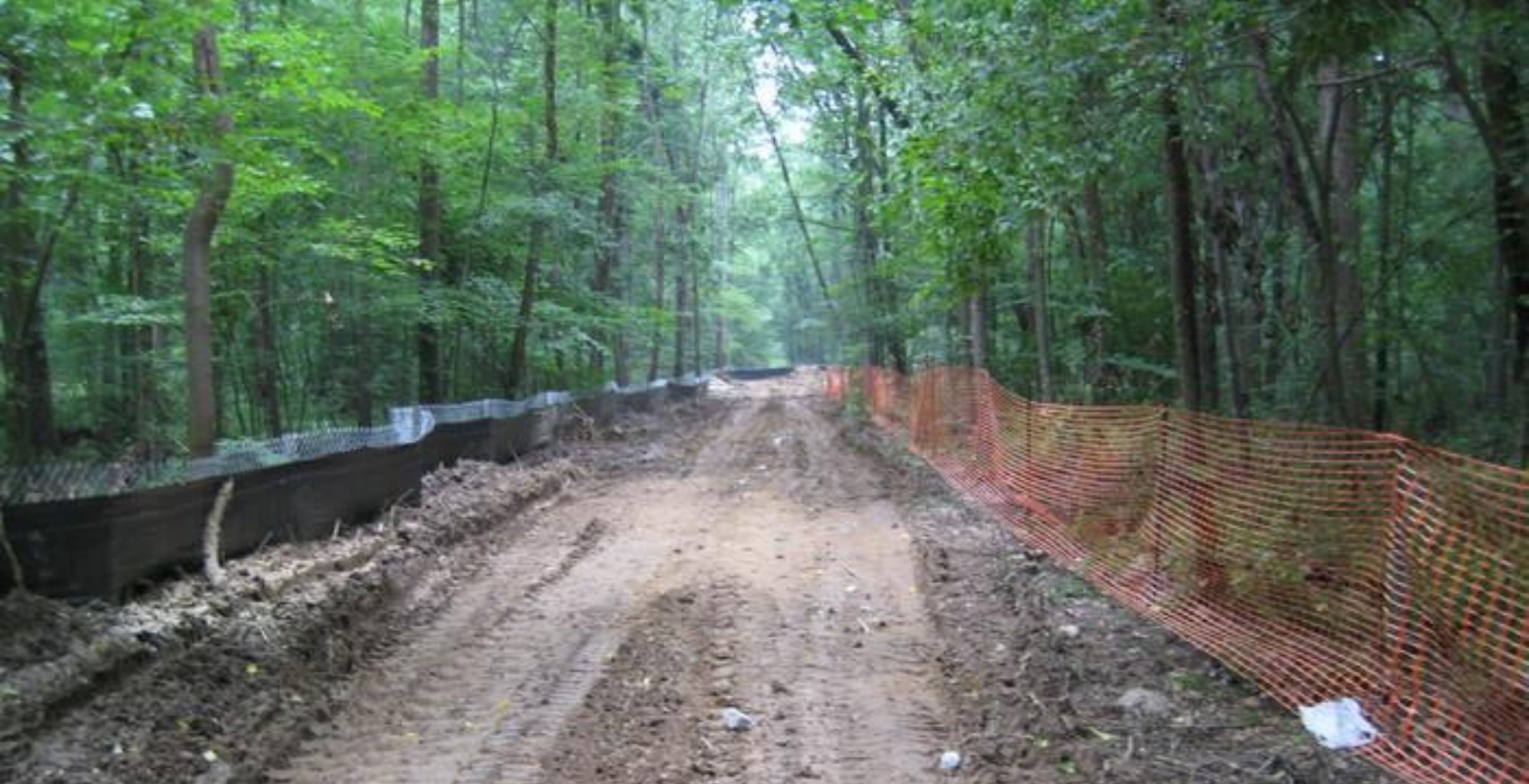
Building of the Cross County Trail, Fairfax County, between tributary crossings ( June 14, 2008 )
