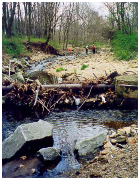
Exposed sanitary pipe running across Little Pimmit Run indicates considerable erosion by the stream.
